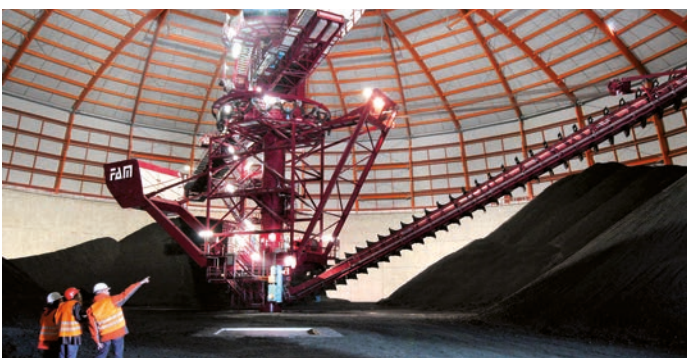
2x circular stacker-reclaimer CST2000/1000.125, coal 2000 t/h - 1000 t/h, Germany
